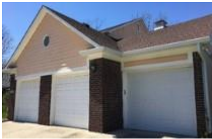
b & c. This garage has a separate door that is more than a 2' plane separation from the other doors.
